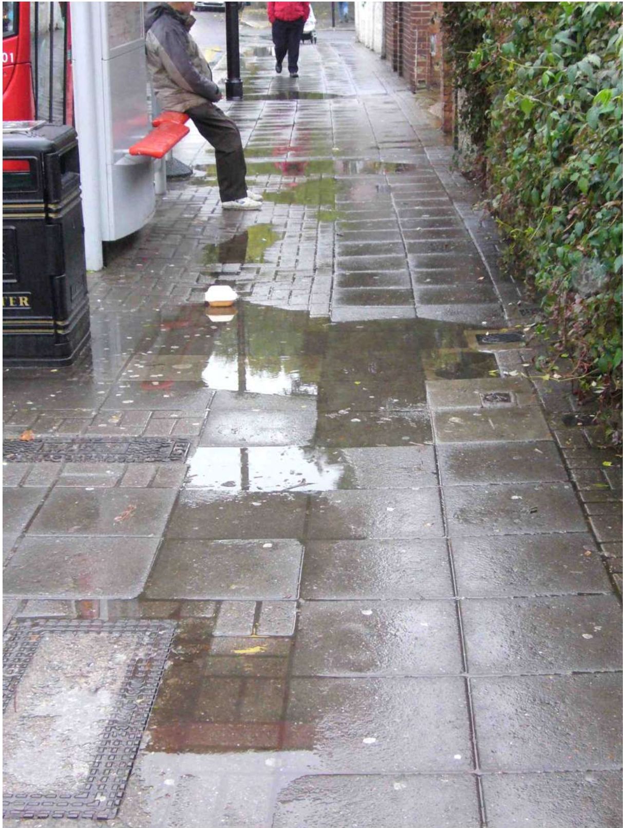
Looking north - puddles at bus shelter (P1060085)
