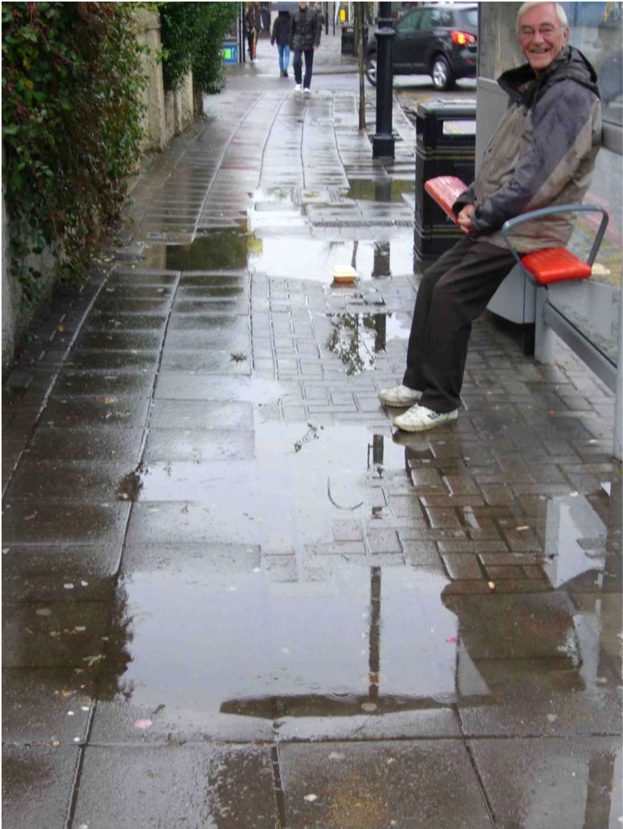
Looking south - puddles at bus shelter (P1060083)
