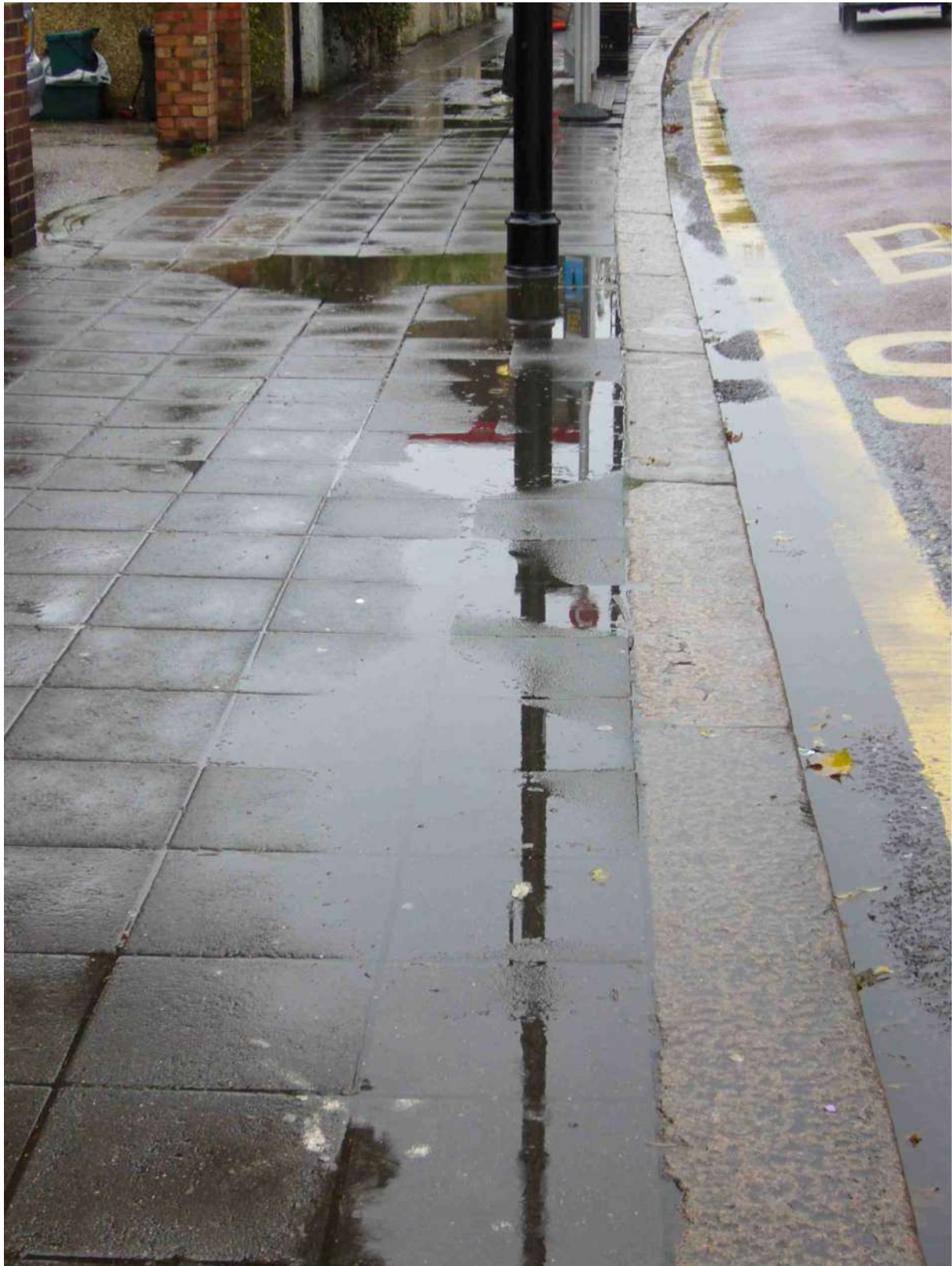
Looking south – puddles around lamppost (P1060082)
